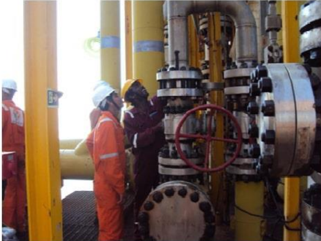
SB MARINE STAFF IN BPA PLATFORM
